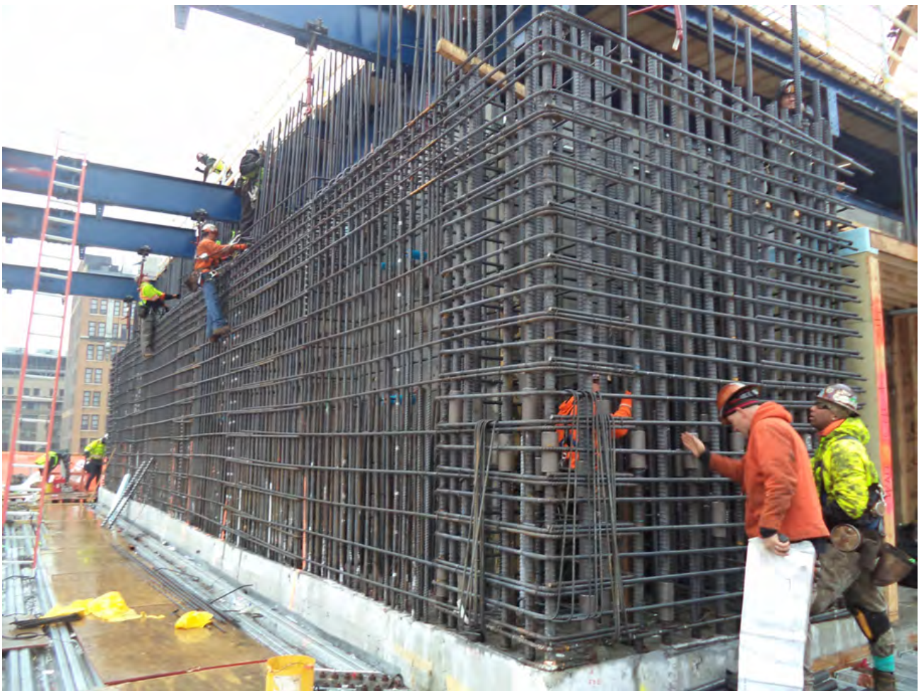
Above: Prefabricated Caisson cages shop fabricated. 12 ea #24 Gr. 80 ksi Multi Bar Caisson
