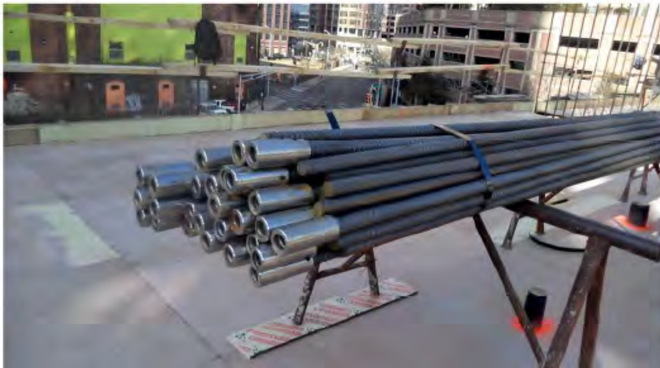
ABOVE: THREADED BARS ARE DELIVERED TO SITE WITH ATTACHED COUPLERS FOR EASIER INSTALLATION
