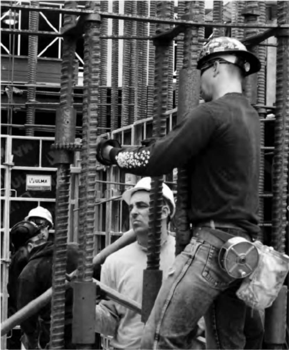
ABOVE: CONTRACTORS THREAD COUPLERS UP TOWARDS UPPER BARS UNTIL MARKINGS ARE EXPOSED
